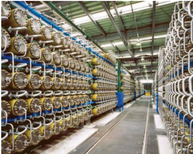
Figure 4.52 High-pressure RO module unit (partial, closeup view).
